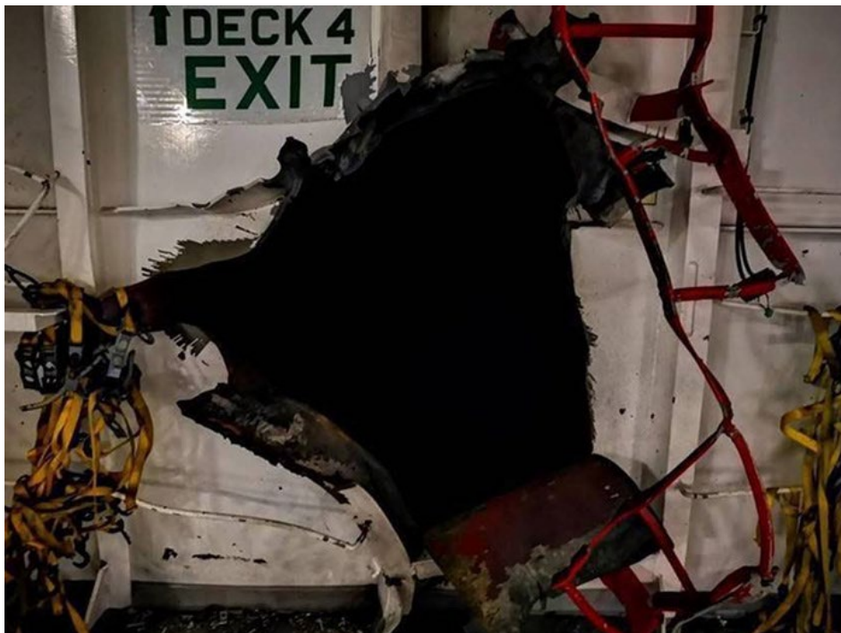
Damage to the Israeli cargo ship HELIOS RAY after explosion (Photo: Channel 13 News)
