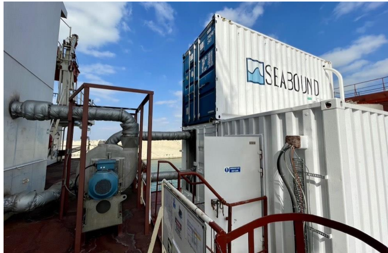
Figure 32 Seabound Installation Onboard
